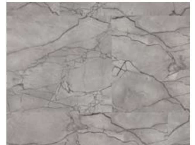
Grey Marble (Installed area) | PL105C | Soft structure
